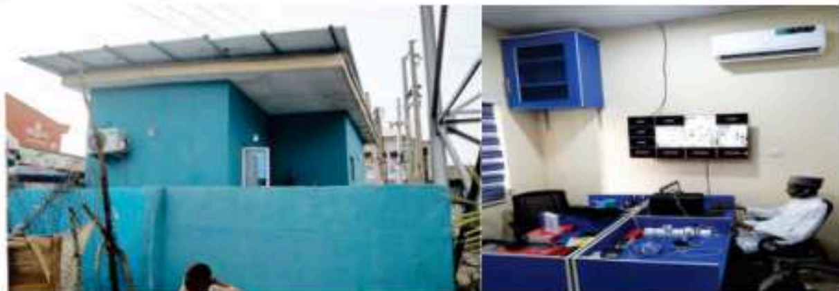
Picture of the Server Room in Gombe Main Market
